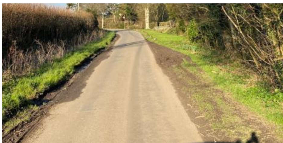
Examples of Damage to Verges
