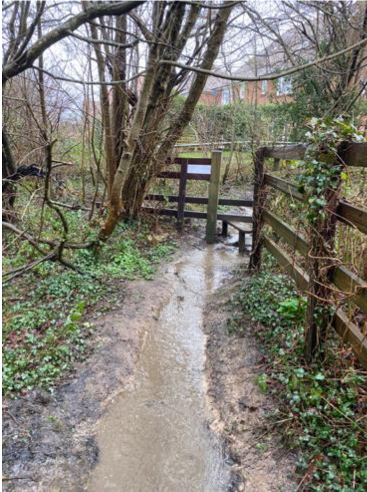
Flooded Public Right of Way below SUDS discharge
