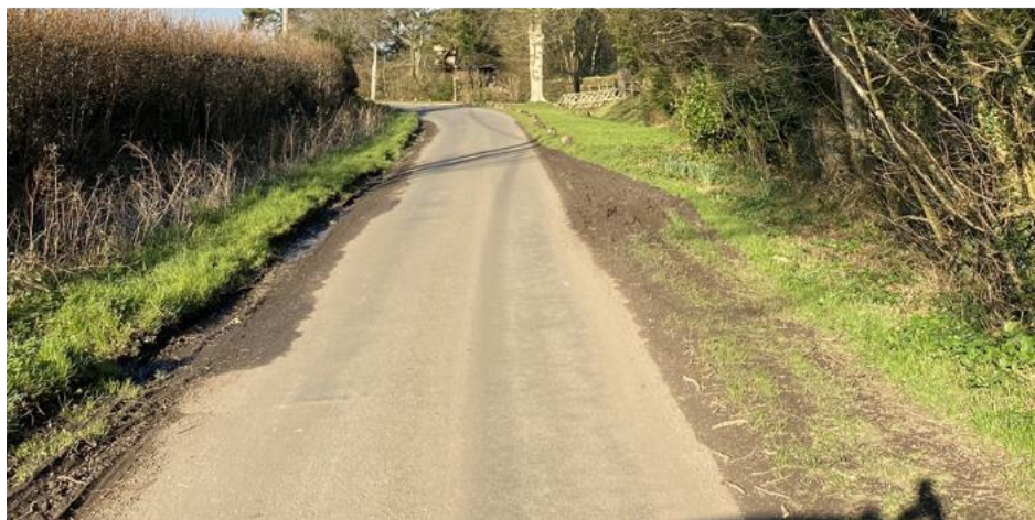
Examples of Damage to Verges
