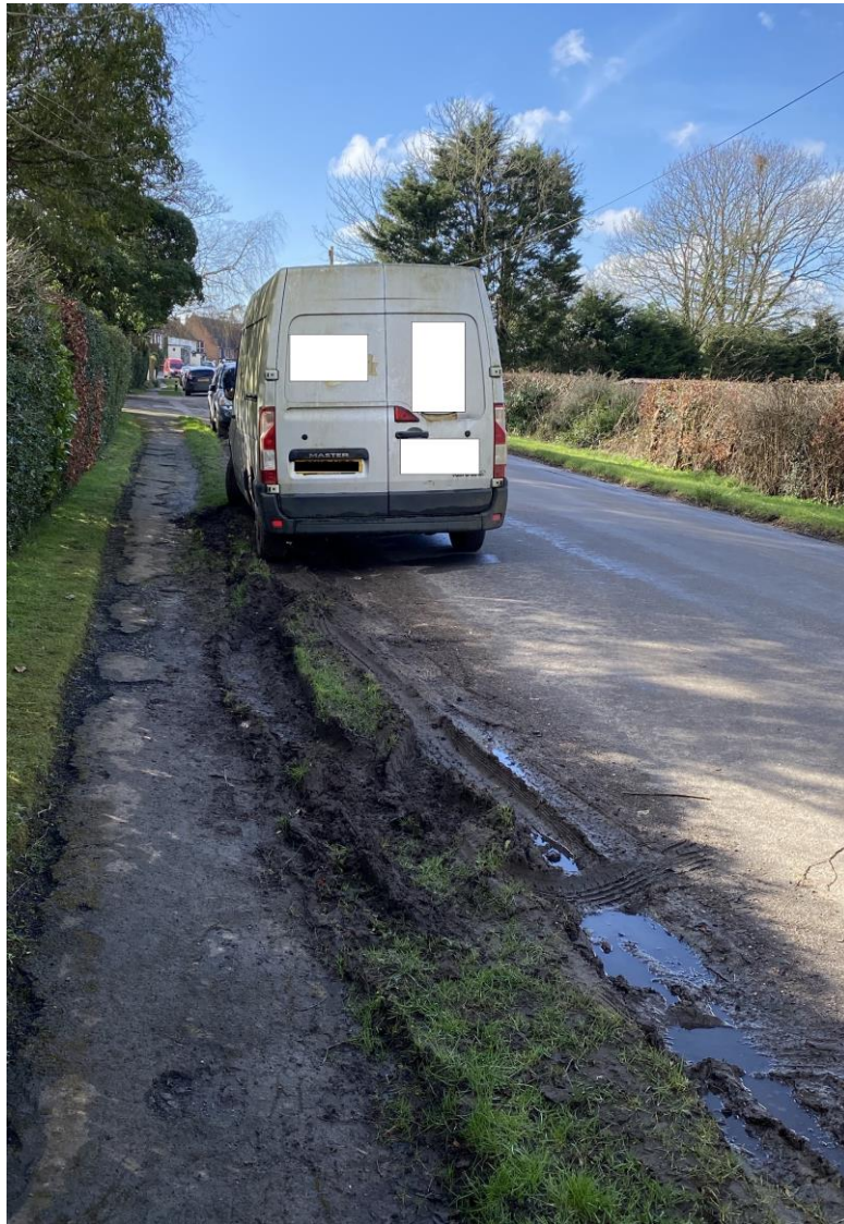
Damage to Verges on Waldron Road
